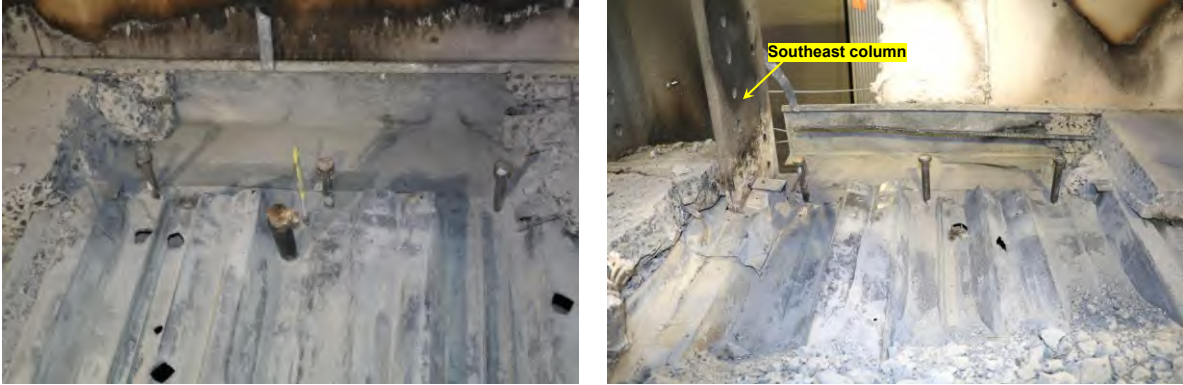
e f Fig. B-23. Post-test photographs of headed stud anchors in the test bay.
